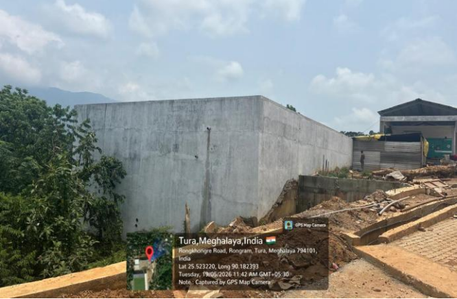
Under Ground Tank
